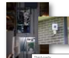
Third-party bridge/access point with patch antenna
