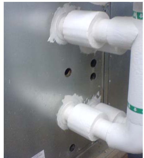
Figure 2. Unsealed coil drain and vent holes.
